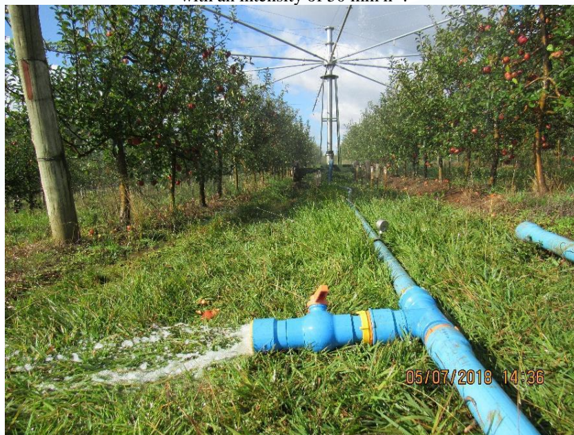
Figure 5: Valve installed to remove water from the system and reduce the flow rate for producing rainfall with an intensity of 50 \text{ mm h}^{-1} .
