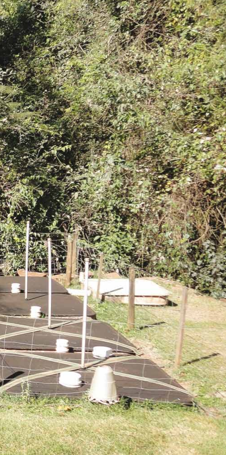
Biodigester septic tank and filter garden
